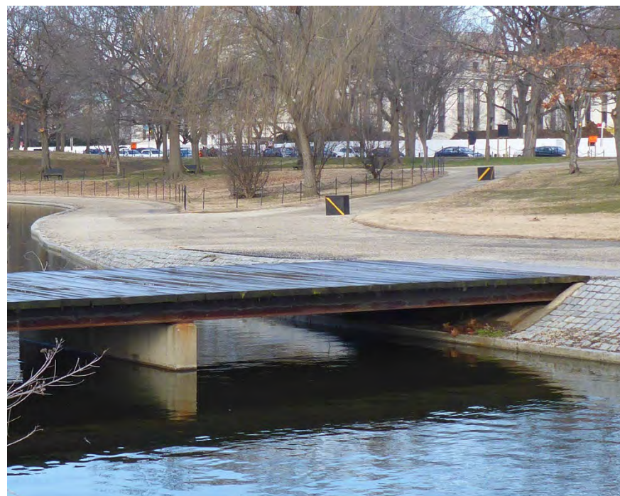
EXISTING, NON-ADA COMPLIANT BRIDGE
