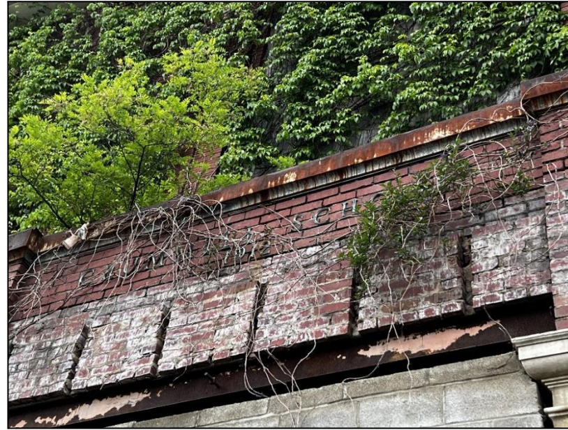
Figure 2: South entrance, missing cornice. Note lettering.
