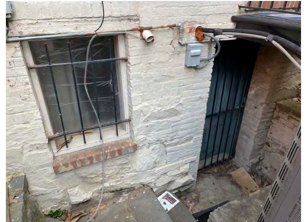
Existing Rear Sub Basement at 2910 M Street, Door Proposed to be removed and inset brick to fill in opening
