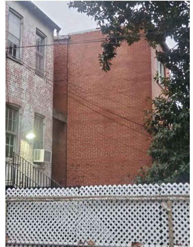
West Elevation of the two-story rear addition (c.1963 – 1960's) show the delineation between the historic rear elevation and the newer construction.
