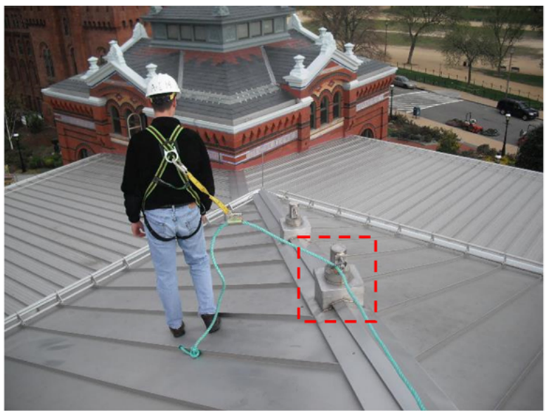
Figure 3.4.7.b – Similar fall protection system installed on the Arts & Industries Building.
