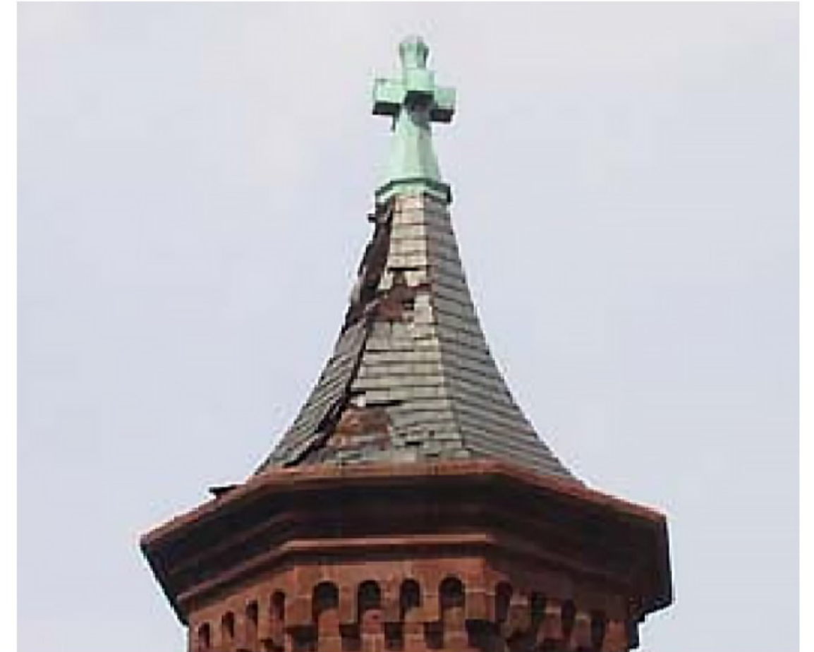
Figure 3.4.6.b – Southeast Tower damaged by a lightning strike in 2005
