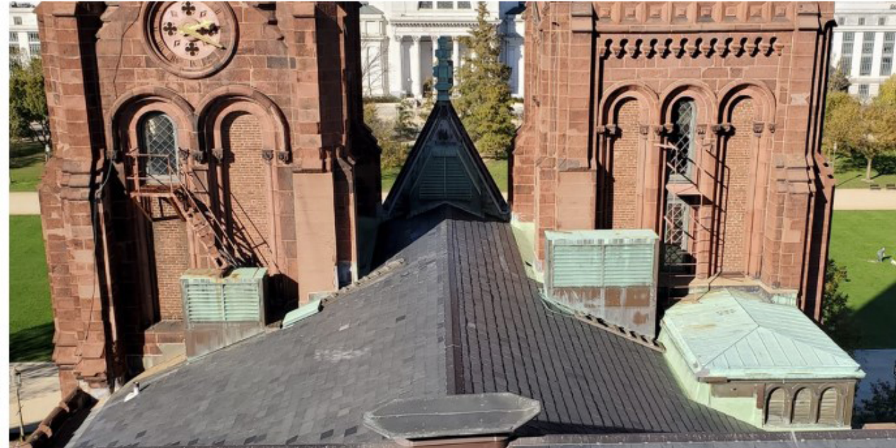
Figure 3.4.7.d – Existing condition of roof access ladder and stairs at the south elevations of the Flag and North Towers
