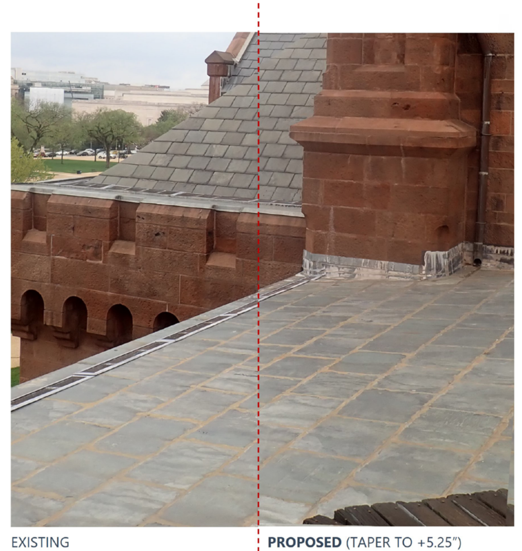
Figure 3.4.3.c – Proposed and existing montage demonstrating the dimensional roof change over the East Range
