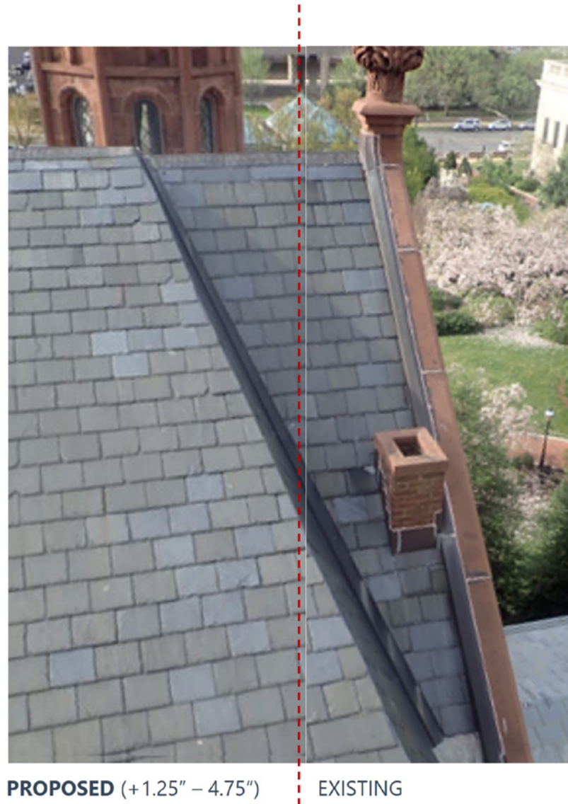
Figure 3.4.3.b – Proposed and existing montage demonstrating the dimensional roof change over the Main Building
