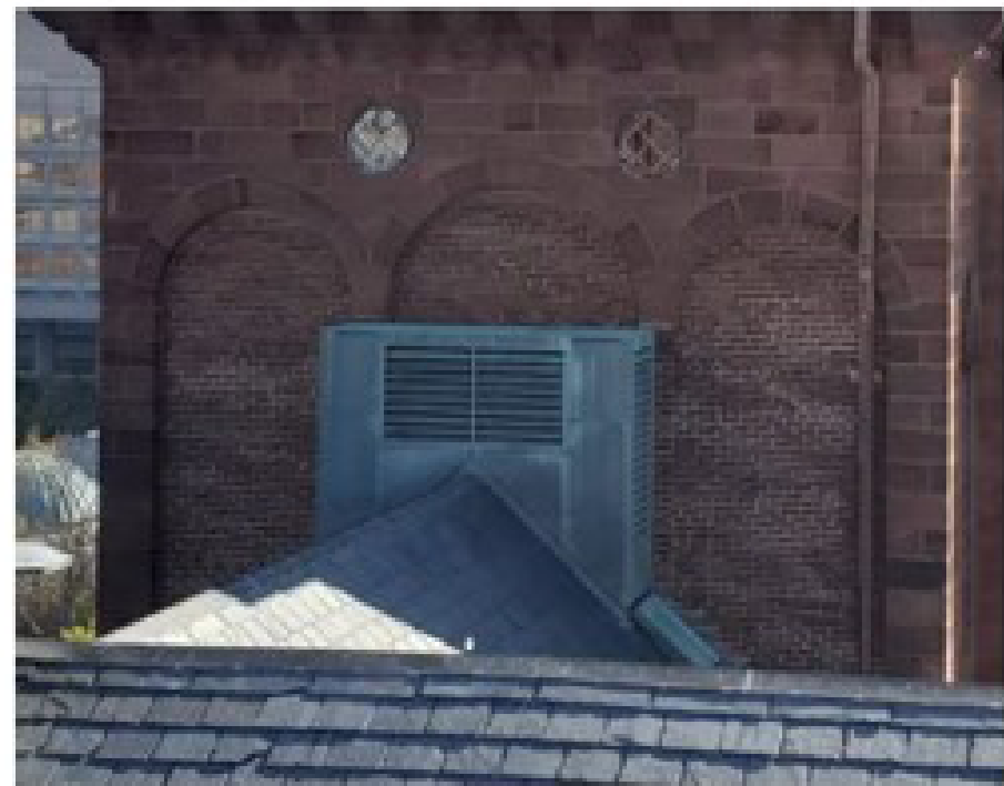
Figure 3.4.1.a - Existing condition of the South Tower peaked roof and mechanical bulkhead to be removed, and the blind arches infilled with brick masonry
