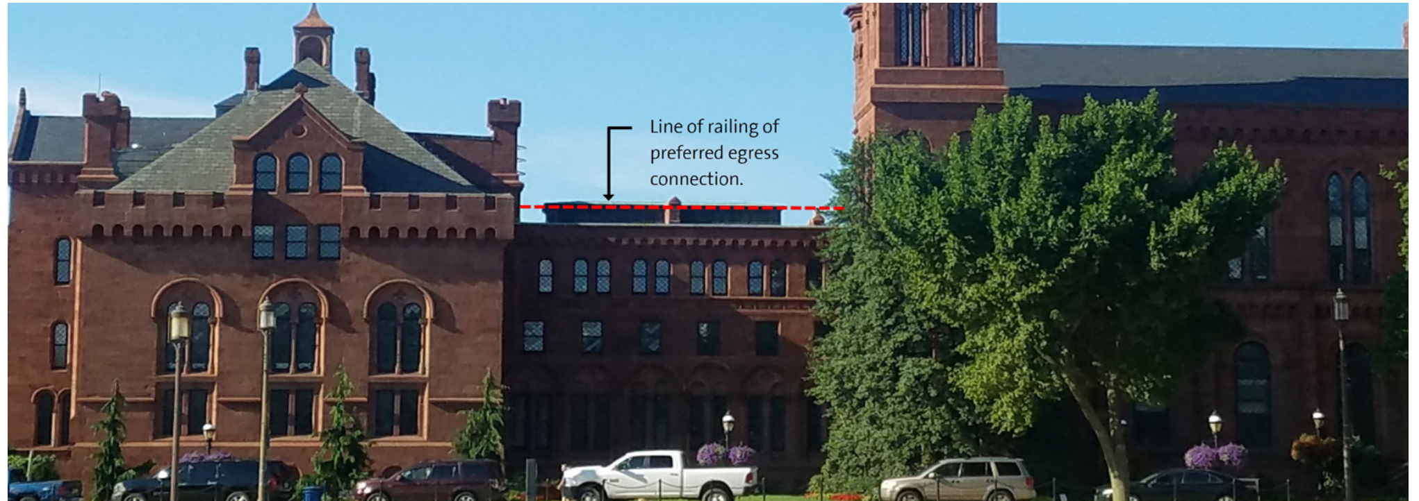
Figure 3.4.5.b – Photograph of the East Range and the visibility of the 1973 mechanical penthouse; red dotted line indicates height of the 42” guardrail
