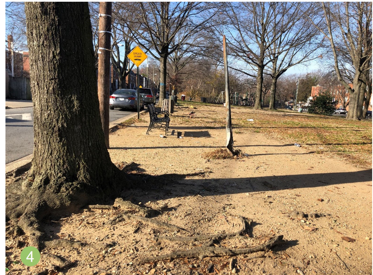
Looking west along Parkland Place, the site has exposed tree roots and lacks groundcover.
