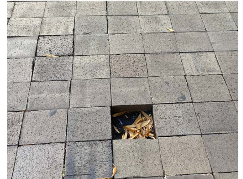
Missing or broken Modernist pavers, bench slats, and other site elements
