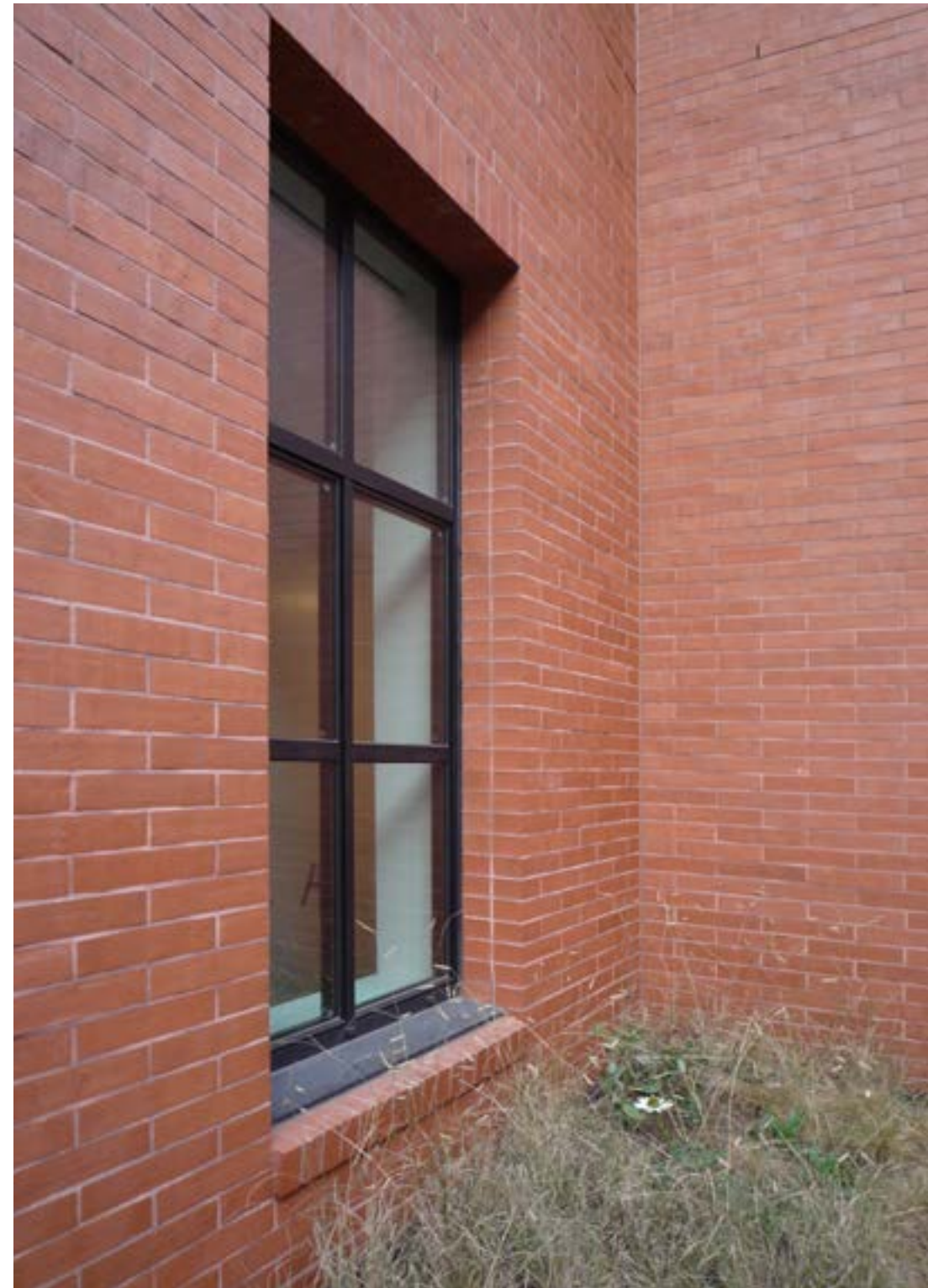
TIGHT BRICK MORTAR JOINTS
