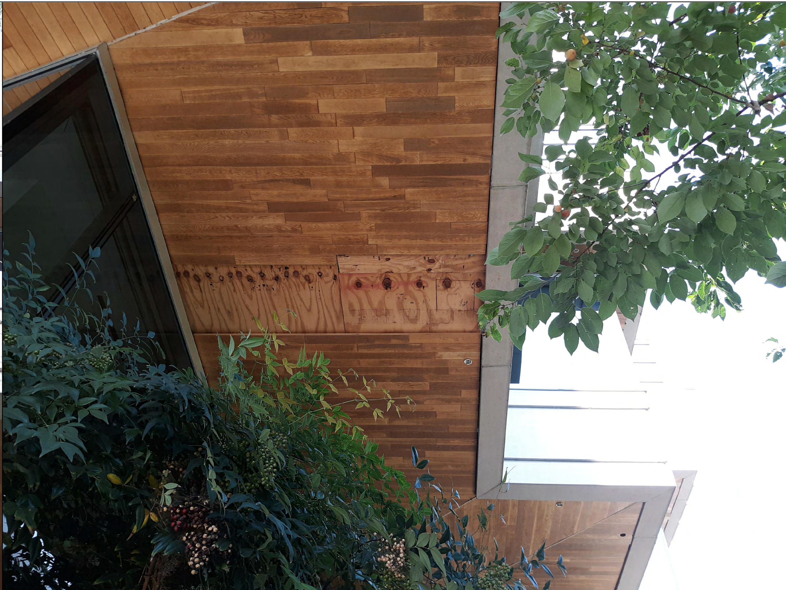
SOFFIT FINISH FALLEN AREA AT EAST SIDE
